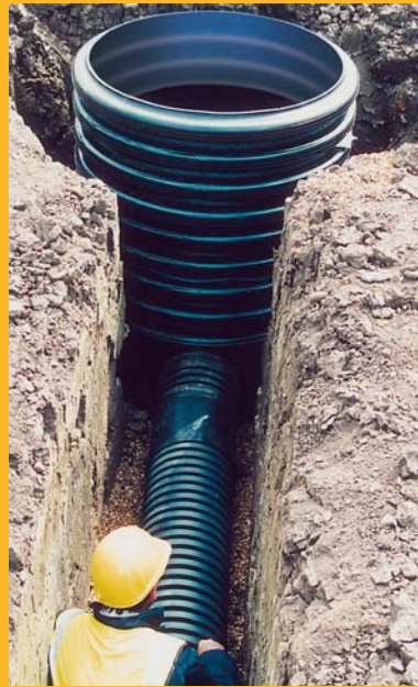
Pipe connected to integral socket on the manhole base
